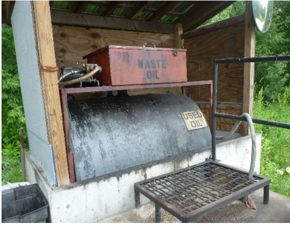
Proper secondary containment for an aboveground storage tank holding used oil outdoors
