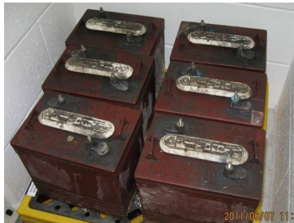
An example of appropriate battery storage: batteries are stored indoors and on an impervious surface.
