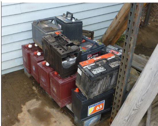
An example of inappropriate battery storage: batteries being stored outdoors with evidence of contact with precipitation.
